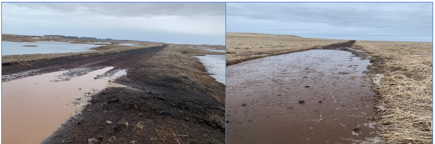
Examples of water pooling and drainage issues on roadways
