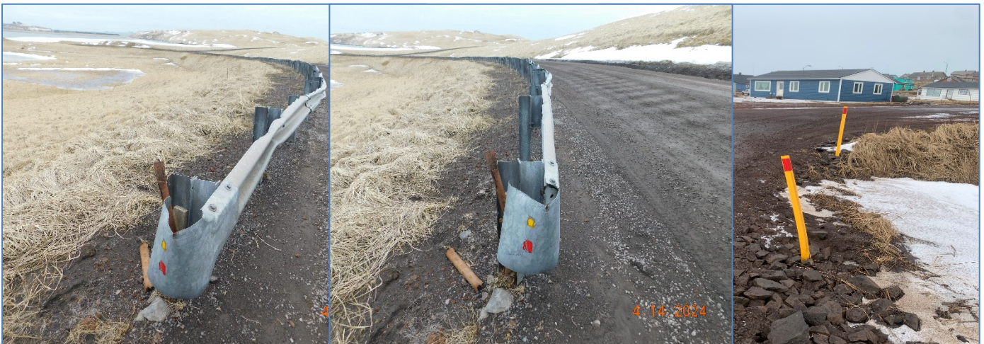
Guardrail conditions on Polovina Turnpike and example of road delineators in Saint Paul
