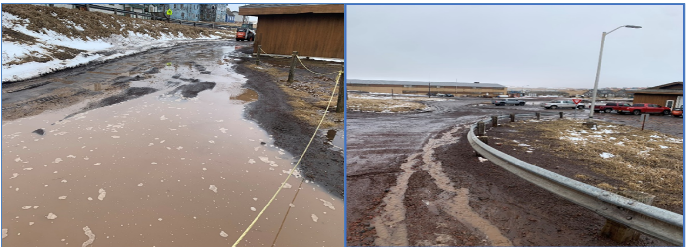
Drainage issues near school access and drop off area at Saint Paul School
